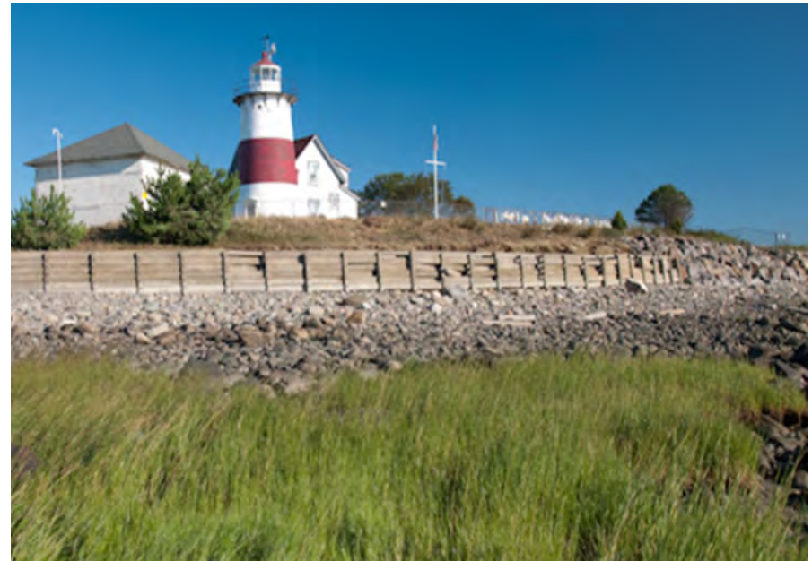
Rip-rap shoreline destroyed by Superstorm Sandy: Stratford example
